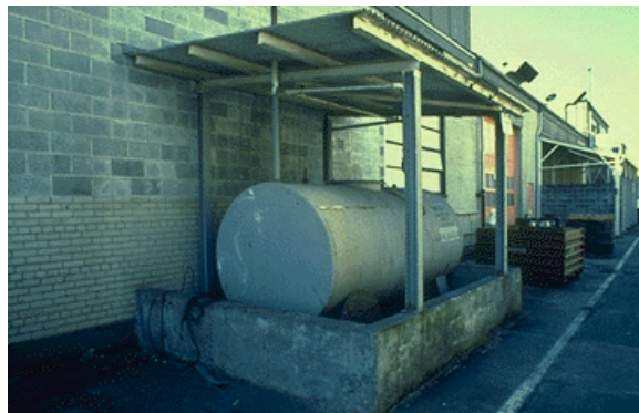
Covered AST with secondary containment
