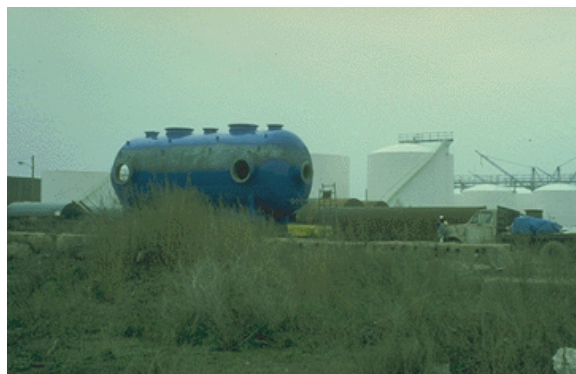
Above ground storage tanks
