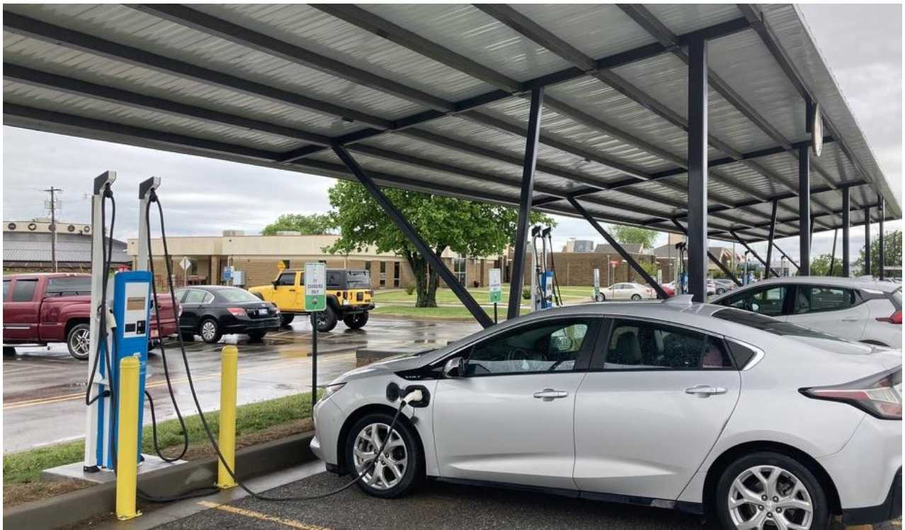
EV Charging Station at the Muscogee Creek Nation’s Tribal Headquarters, Tulsa, Oklahoma. Photo by Andy Bessler
