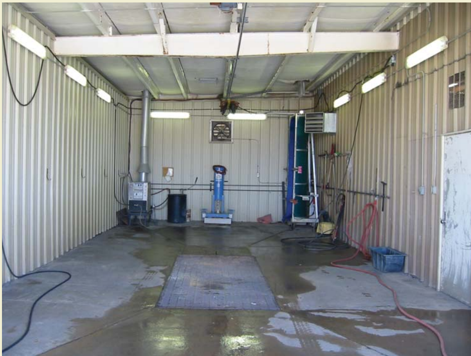
Floor drains in service bays might lead to a Class V (Five) Motor Vehicle Waste Disposal Well.
