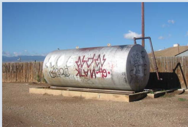
Wrong: This AST has inadequate secondary containment, and no way to prevent vehicles from hitting it.
