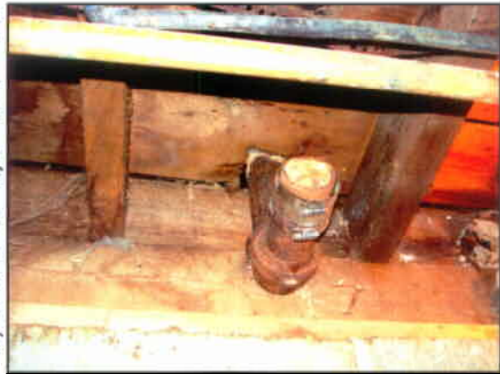
Evidence of mold during walk-through of vacant residence.
