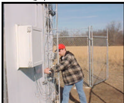
Frank Geasland, Air Quality Specialist, Quapaw Tribe, Oklahoma, erecting a Meteorological Tower.
