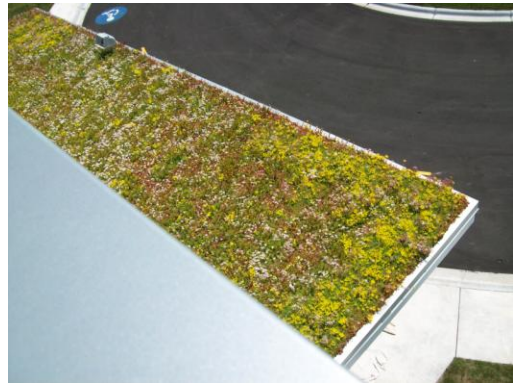
A roof with growing vegetation is one of the many green features of the Resource Management Division building.
