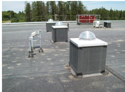
Light collectors on the roof bring natural light into the Resource Management Division building.
