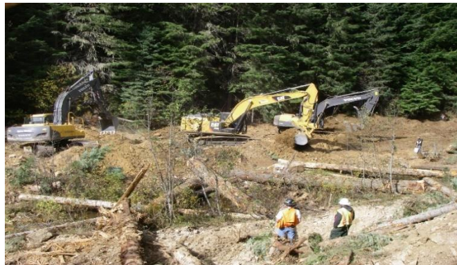
Fish passage dam removal and large woody debris (LWD) re-introduction in critical bull trout (endangered species) habitat area along the St. Joe River in North Idaho. USFS as Lead Trustee.
