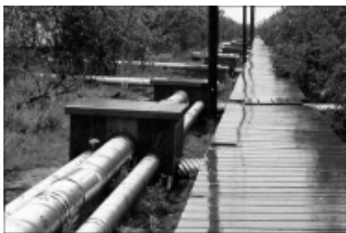
Piped water system.
