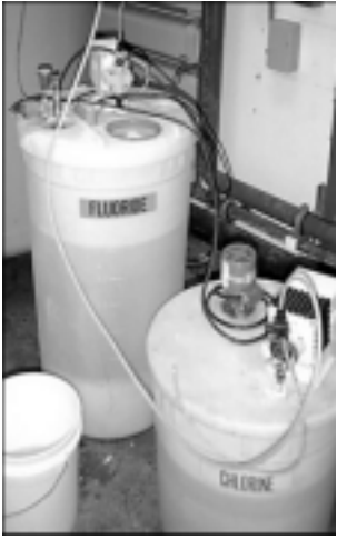
A water treatment system that adds chlorine and fluoride.
