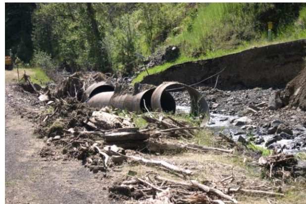
Figure 22. Culvert and stream damage after a flash flood, 2010. Photo: Casey McCormack.
