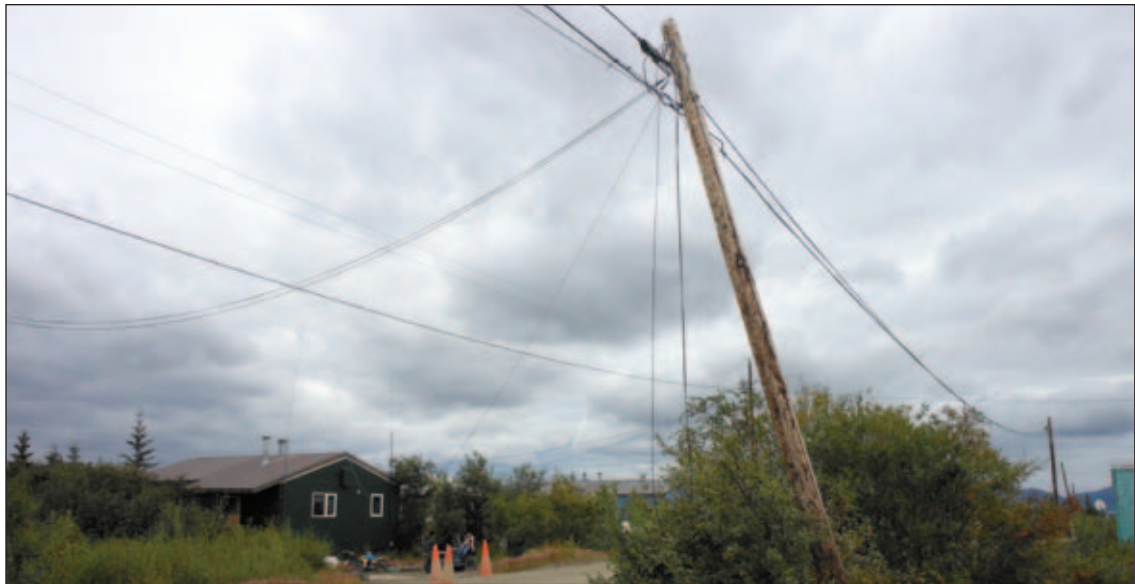
Leaning utility poles are a safety concern. Mike Brubaker, 2011.
