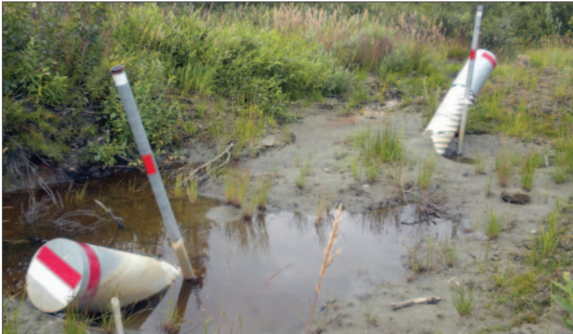
Sagging sewer main clean outs. Mike Brubaker, 2011.
