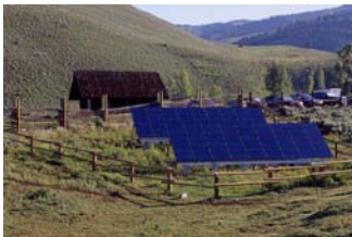
Solar panels and propane generator at Yellowstone National Park; National Park Service photo.
