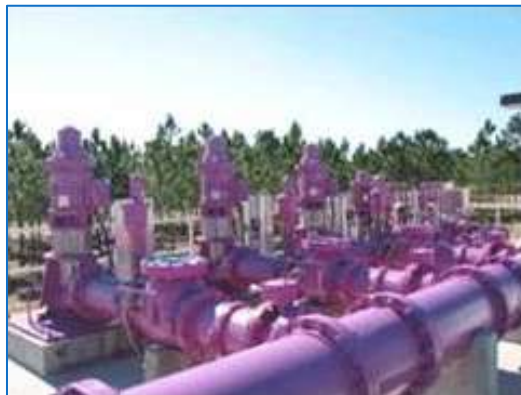
Figure 63 - Piping used for distribution of reclaimed wastewater is colored purple to distinguish it from potable water pipes. (SFWMD)
