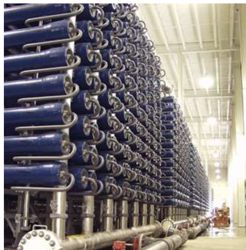
Figure 53 - A modern large scale reverse osmosis installation
