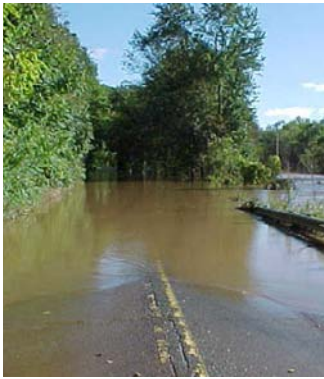
Damage from Hurricane Ivan at Delaware Water Gap National Recreation Area; NPS photos.
