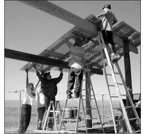
NAPV Installs Panels on the The Seba Dalkai School on the Navajo Nation. Photo credit: NAPV
