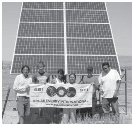
Honor the Earth and Solar Energy International solar installation in Skull Valley
