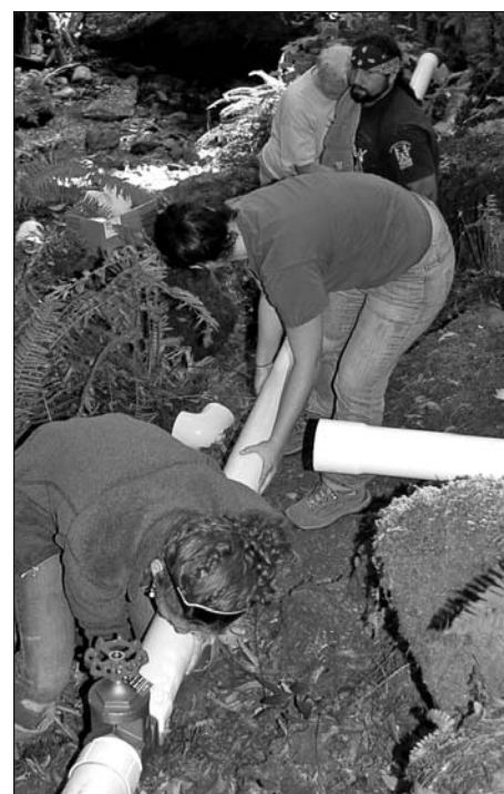
Micro hydro installation. Photos courtesy Sustainable Nations
