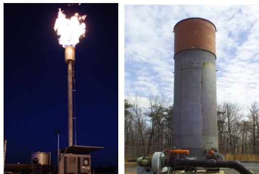
Figure 1-4. Open (left) and Enclosed (right) Flares
