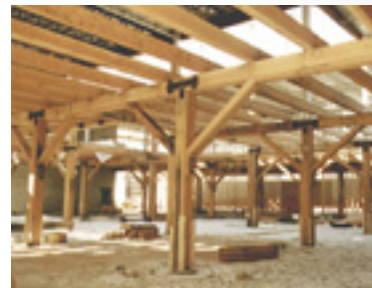
Douglas Fir from St. Lawrence River were reused as columns and beams in the Ottawa store.
