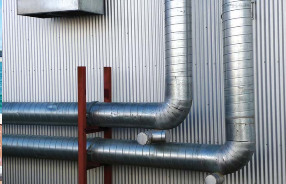
District heating system in Iqaluit, Nunavut
