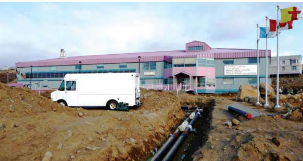
Underground Pipes Carrying Heat from Iqaluit Generating Station Photo by: Daniel Van Vliet
