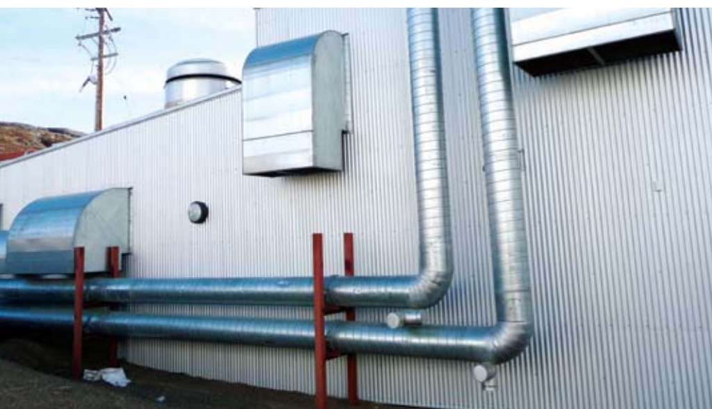
Insulated Pipes Providing Heat to a Community Building in Iqaluit Photo by: Daniel Van Vliet
