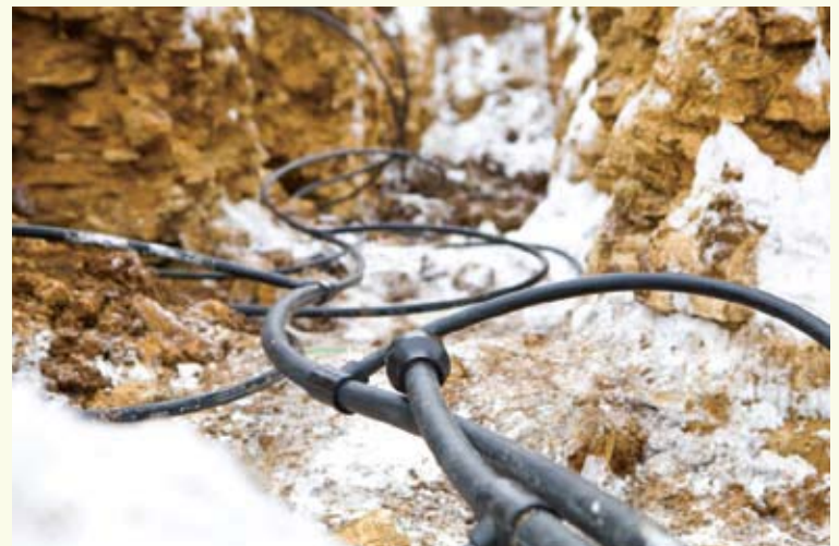
Ground Source Heat Pump Coils
