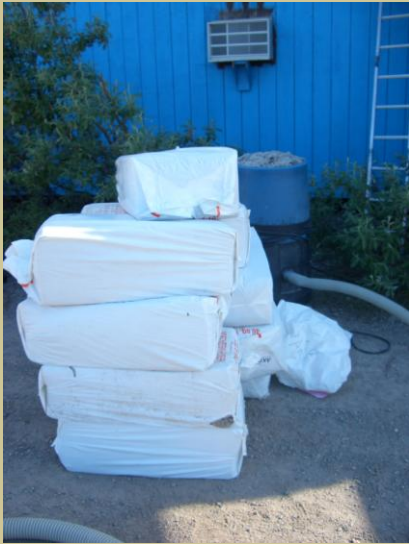
Cellulose insulation added to the village store in Anaktuvuk Pass to improve heating efficiency.
