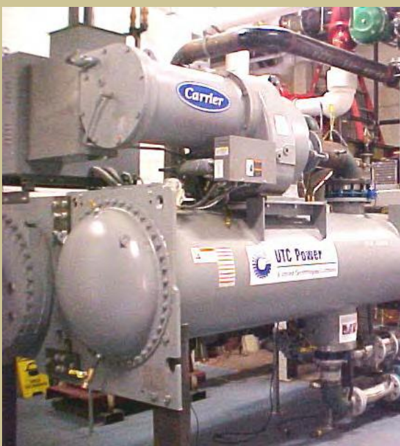
The pump and generator unit for the Chena Hot Springs geothermal power plant
