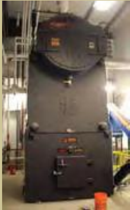
Wood chip burner in Tok Photo from Alaska Energy Authority 2011 Renewable Energy Atlas
