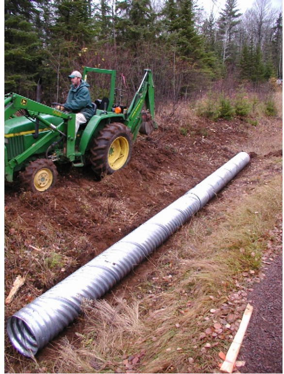
Some storm sewers are made of galvanized steel. You may see the sewer pipe at the outfall to a ditch or water body. You may also see the pipe where it leads into catch-basins. The appearance of metal and spiral construction is an indication. Pipes with parallel ribbing are of PVC or other materials.
