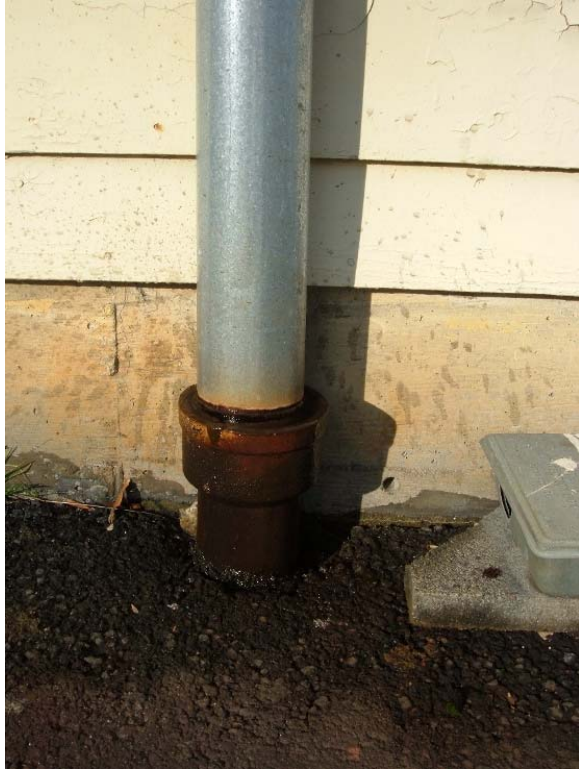
Some downspouts are made of galvanized steel. They can contribute significant amounts of zinc in the discharged stormwater.
