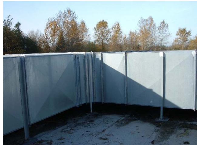
Galvanized HVAC or other ductwork on facility roofs is a common source of zinc in runoff.
