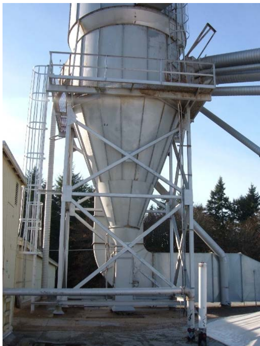
Roof-mounted air-pollution scrubbers may have large surfaces of galvanized metals
