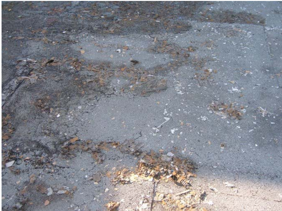
Debris on the ground, such as dust, sawdust, dry leaves, or bark dust, may soak up oil and/or hydraulic fluid. These can become a major source of zinc with rainfall and runoff. Sweeping with vacuum sweepers removes the large and small particles, in some cases greatly reducing zinc in runoff.
