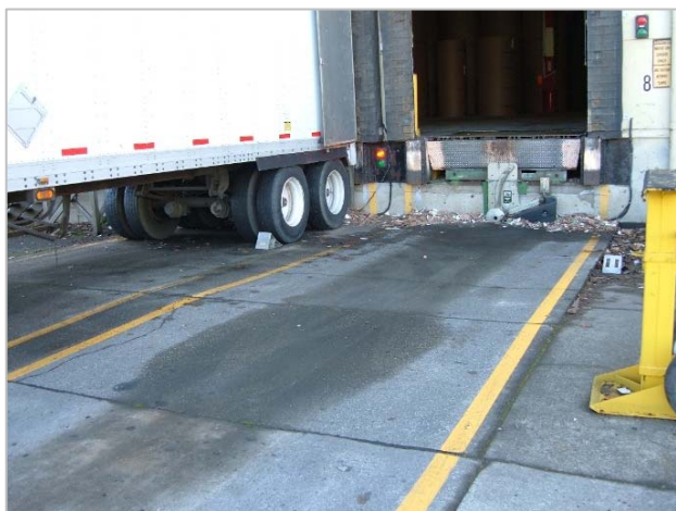
Motor oil on pavement at loading dock. If the pavement has few loose particles (if it is fairly clean other than oil and hydraulic fluid spots, you may need to pressure wash with vacuum pickup.
