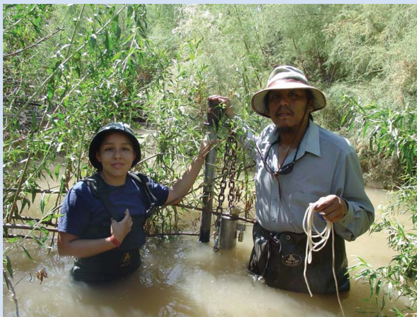
Gila River Indian Community YSI Sonde installation for continuous water quality monitoring at the Pee Posh Wetlands. Photo courtesy of Gila River Indian Community.
