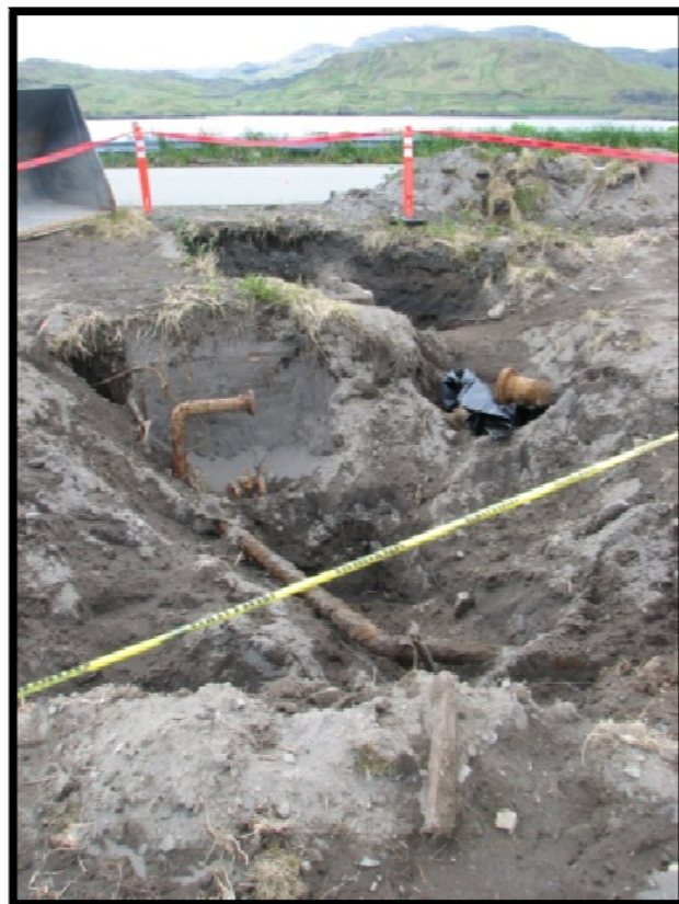
Adak's abandoned pipelines
