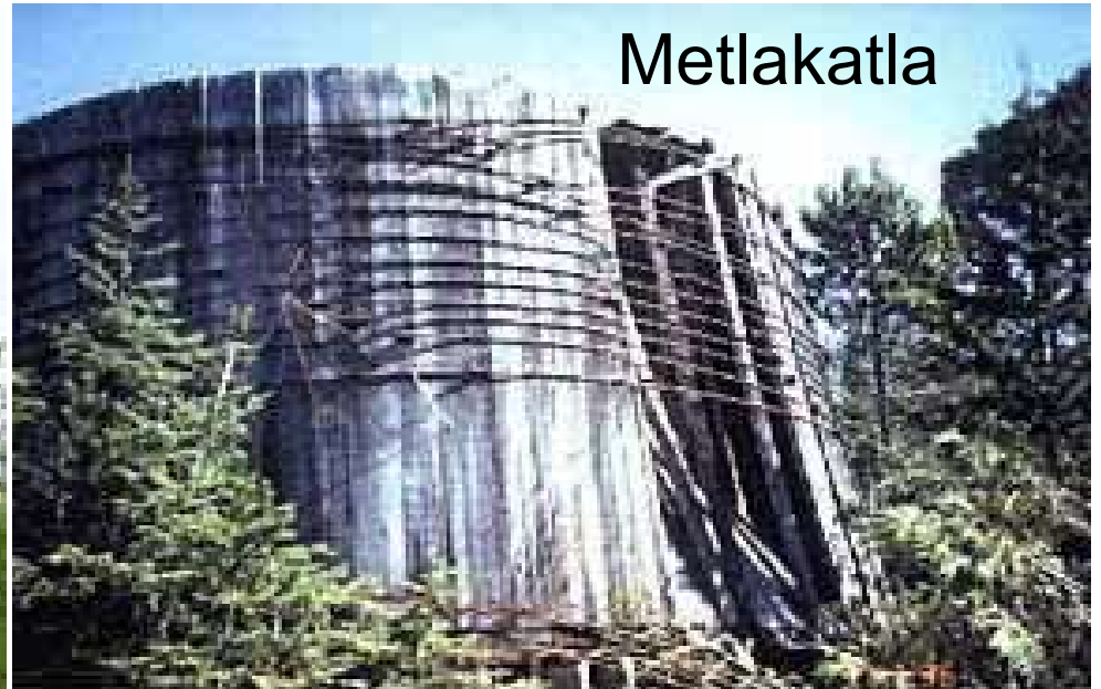
Prominent odor and distressed vegetation surround three collapsed 80,000 gallon fuel storage tanks.
