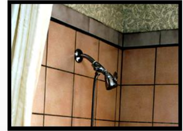
Mold on grout. Photo courtesy of EPA
