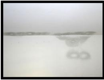
Water stains on wall and ceiling. Photo courtesy of EPA
