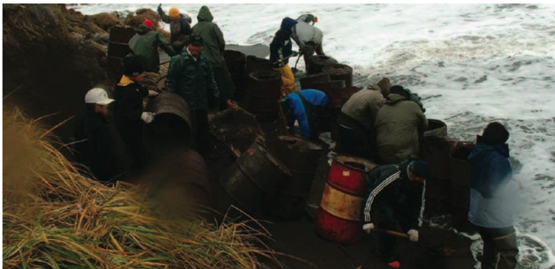
Emergency erosion control on the coastline near Kivalina, AK. Photo courtesy Millie Hawley.
